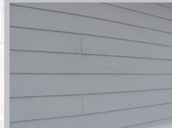
Discolored finish at Unit 200
