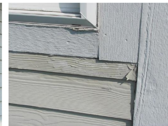
Peeling paint finish at Unit 300
