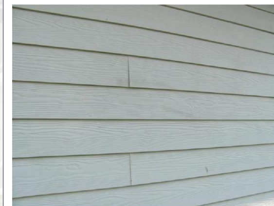
Discolored finish at Unit 200
