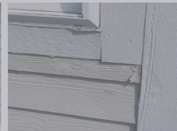
Peeling paint finish at Unit 300
