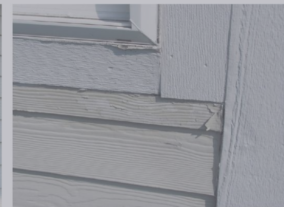
Peeling paint finish at Unit 300
