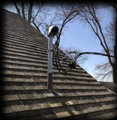
Electrical Meter Mast: Provide electricity to older homes.
