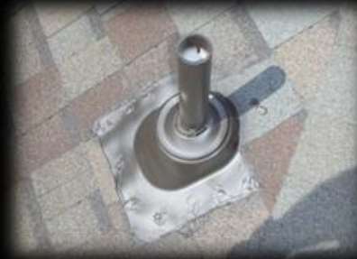
Pipe Jacks: Plumbing vents to allow air to enter the drainage system.
